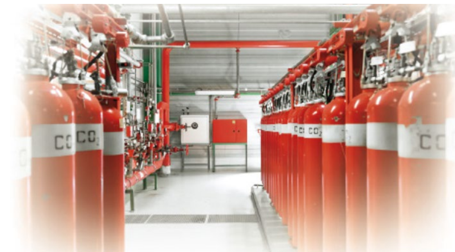
Figure 45: Fixed gas extinguishing system.
