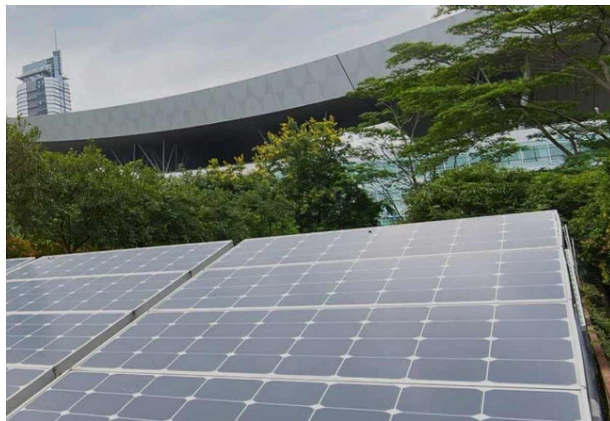
Figure 14: On-site photovoltaic generation of renewable electricity.
