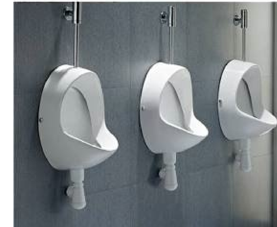
Figure 23: Urinals can be more water efficient if controlled by presence sensors.
