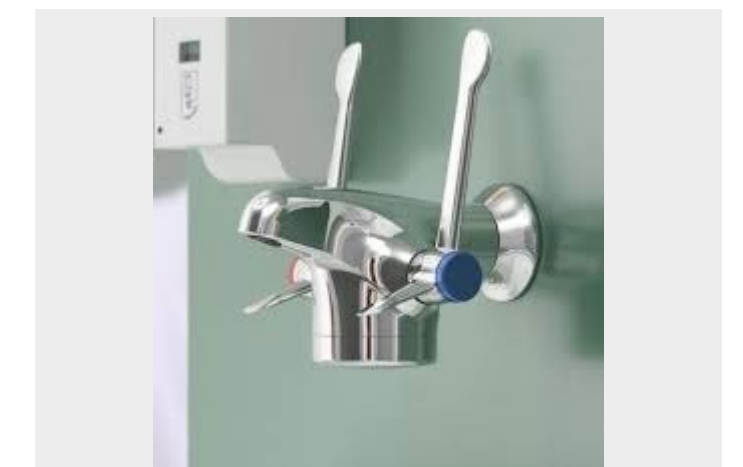
Figure 6: Domestic hot water sinks are common in all healthcare areas.
